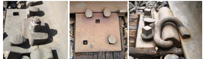
Figure 2: Rail Restraint Methods, Left to Right: Curve Blocks, Cut Spikes in 8- by 18-inch Tie Plates, and Elastic Fasteners
