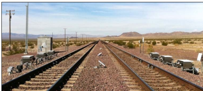
Figure 1. Two TBOGI-HD Detectors on Double-Track
