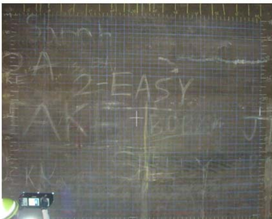
Figure 2: Grid Lines applied to Tunnel Lining Wall to assist in detailed inspection of the Thermal Anomaly found in Figure 1.
