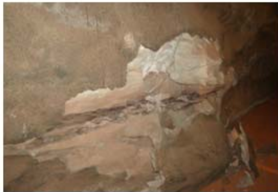
Figure 5: Shotcrete Lining Failure
