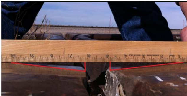
Figure 1. Longitudinal Profile of a Worn Flangeway Corner
