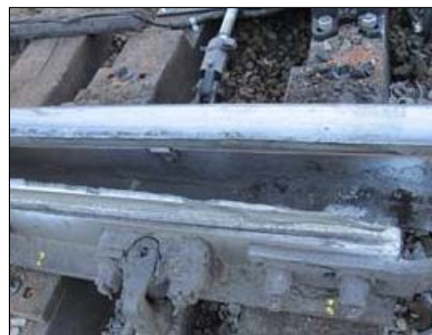
Figure 1. Switch Point Damage
