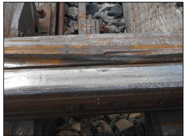
Figure 8. Metal Flow and Wear on Lateral Guard of Right Switch Point at 36–42 inches from POS
