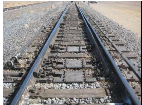
Figure 10. Conventional Split Switch Turnout at FAST
