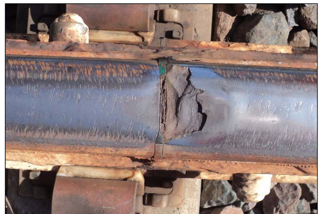
Figure 2. Severe Rail-End Batter at the Joint
