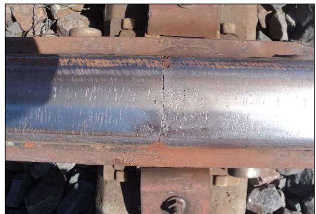
Figure 1. Severe Metal Flow developing over the End Post
