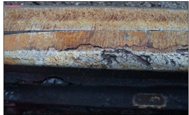
Figure 4. Severe Spalling on the Gage Side of the Taper Cut IJ
