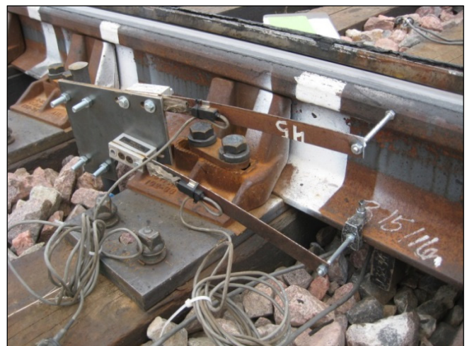
Figure 5. Bending Beams (Displacement Transducers) in Place to Measure Dynamic Lateral Railhead and Base Displacement under Traffic
