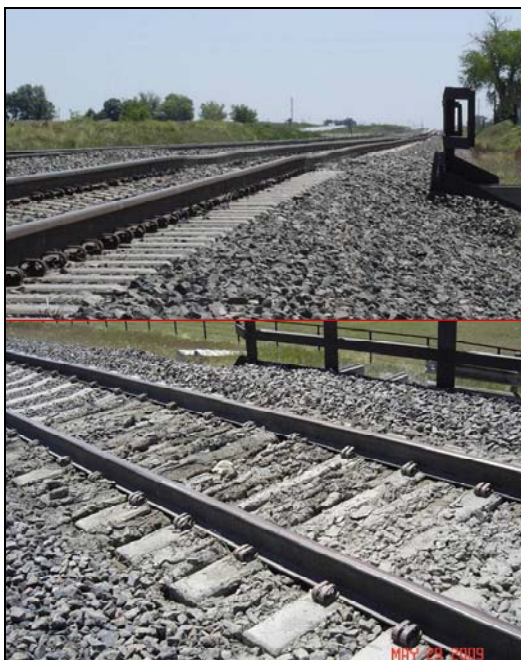
Figure 1. Rough Track Geometry and Mud Pumping Associated with Bridge Approaches
