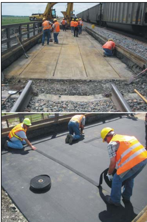
Figure 4. Ballast Mats for a Bridge at Western Mega Site
