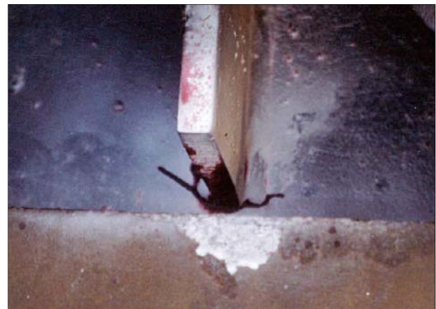
Figure 2: Web Crack beneath Intermediate Stiffener Just Above Tension Flange
