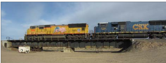
Figure 1: Steel Bridge at FAST with 65-foot Welded Deck Plate Girder Span (left) and 55.5-foot Riveted Deck Plate Girder Span (right)
