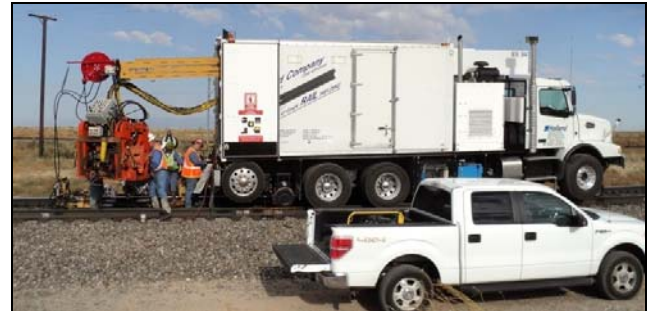
Figure 1. Holland Mobile HDR Weld Truck on Track and being prepared for Welding
