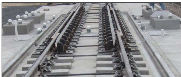
Figure 1. Gage Widened Section with Guardrail and Expanded Flangeway Clearance for Holding Ultrasonic Probes
