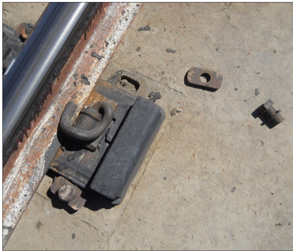
Figure 3. Direct Fixation Slab Track showing Broken Anchor Bolt
