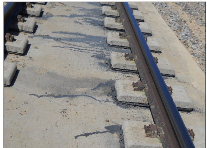
Figure 2. Independent Dual Block Tie Slab Track showing Deterioration of Rubber Boots around Rail Seat Blocks
