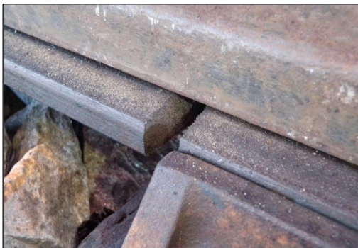
Figure 6. Base Corner Defect found in VAS-2 High Rail Field Side Base Corner on Base Plate Corner Mating Surface
