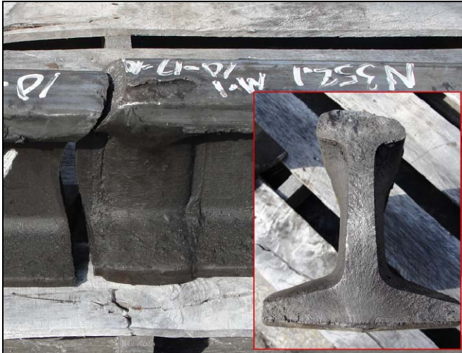
Figure 6. WGW O6 with Shelling on Gage Corner and Fatigue Fracture from Base of Weld — Inset Shows Fracture Face — Fatigue Initiated at Runout at Base of Weld
