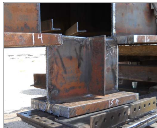
Figure 2. Sample Removed for Fractographic Analysis of Major Crack
