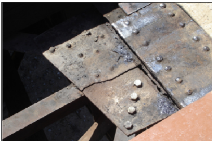
Figure 6. Top Gusset Plate Defects in 55.5-foot Riveted Girder Span at FAST
