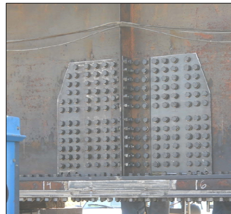
Figure 3. Repair Installed on Web and Tension Flange of 65-foot Welded Girder Span
