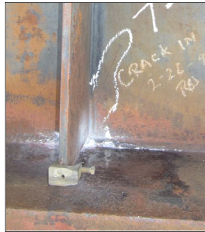
Figure 1. New 8-inch Crack in Web and Tension Flange of 65-foot Welded Girder Span
