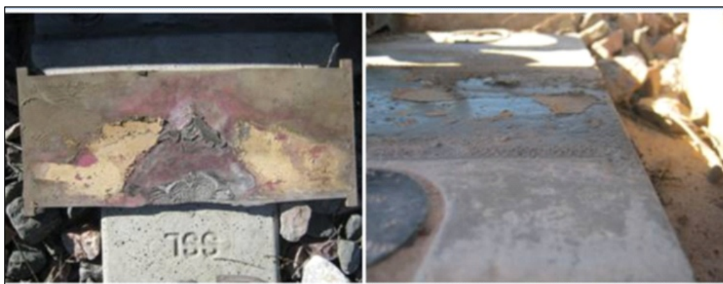
Figure 3. Tie and Pad Deterioration on Half-Frame Tie
