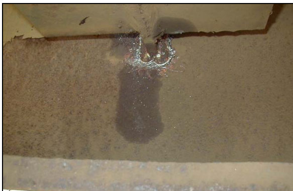
Figure 5. Treated Weld Detail
