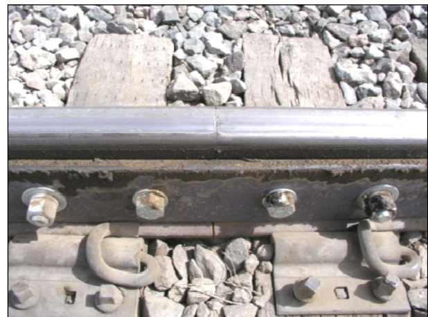
Figure 7. A Standard Rail Joint in Track
