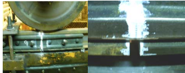
Figure 1. Rail Joint in RLM (left); Notch in the Bottom of Joint Bar (right)
