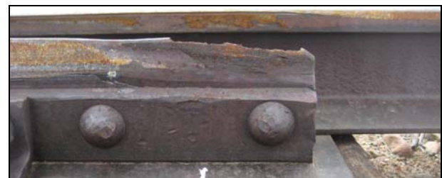
Figure 4. Four-inch Chip Broken off a Switch Point
