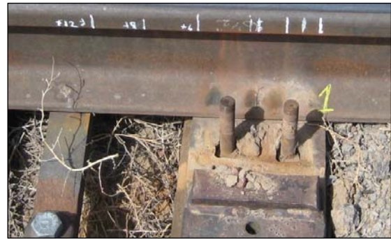
Figure 8. Chair Brace Missing (No. 1 at POS)
