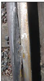
Figure 6. Crushed Wing Rail
