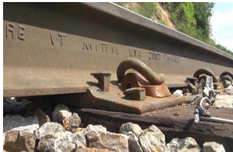
Figure 3. 18-inch Tie Plates and Elastic Fasteners
