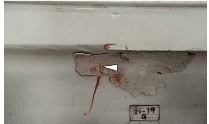
Figure 4. Magnetic Particle Inspection of Crack under Railhead (Arrow indicates location of crack initiation behind flashing under the railhead.)
