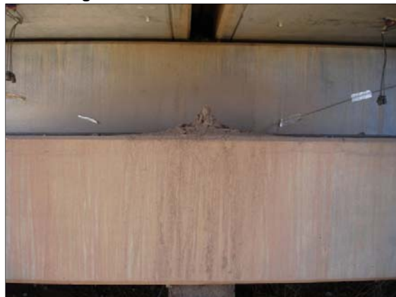
Figure 7. Evidence of Fouled Ballast
