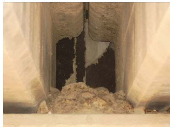
Figure 6. Evidence of Fouled Ballast
