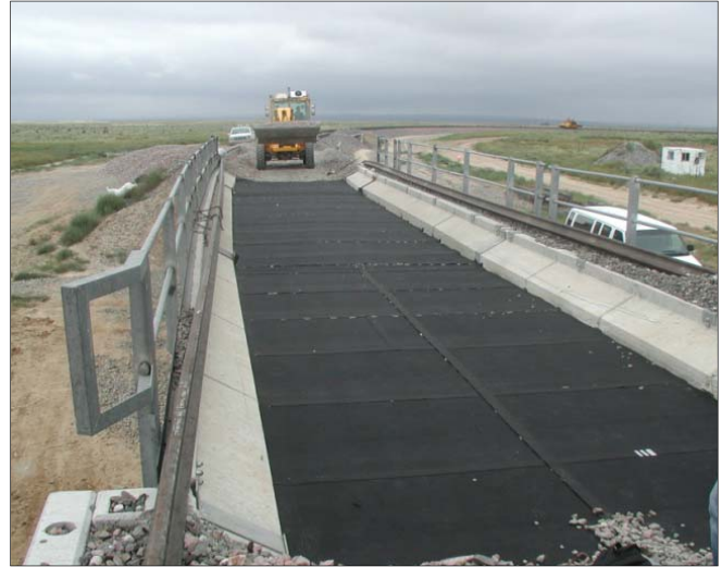
Figure 1. Getzner Ballast Mat on SOA Bridge
