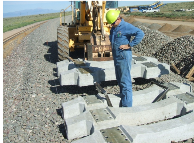
Figure 1. Half-frame Ties in Test at FAST
