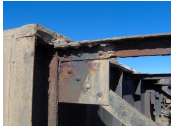
Figure 2a. Pre-existing Rusted Member
