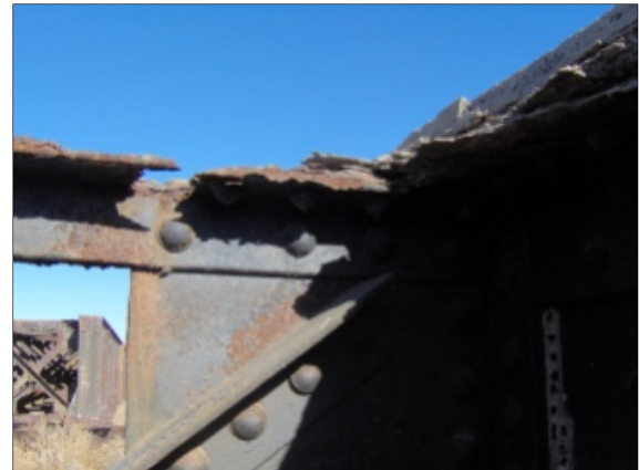
Figure 2b. Pre-existing Rusted Member
