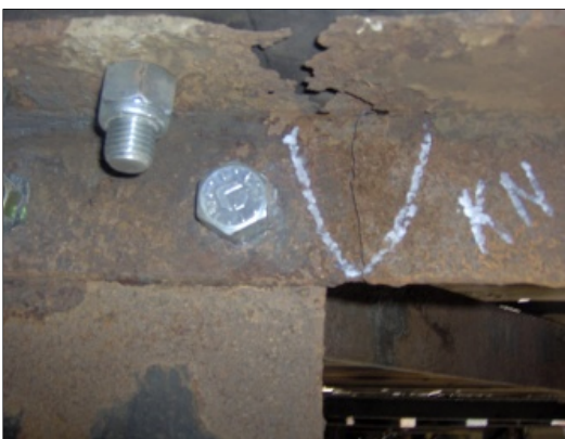
Figure 4a. Cracked Lateral Bracing Member
