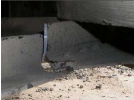
Figure 3a. Broken Member
