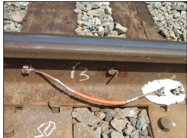
Figure 6. Replacement Wire Connection (Left) and Original Damaged Rail Attachment (Middle) after Passage of a Ballast Regulator
