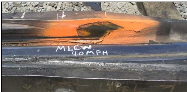
Figure 4. Back of Wheel Impact Location on the Flair of the Frog Guard while running on the Main Line at 40 mph in Trailing Point Direction
