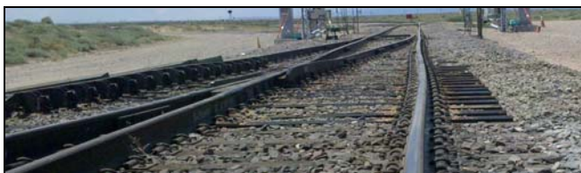
Figure 2. Lateral Misalignment in the Area of the Partial Flange Bearing Frog from HAL Train Operations on the HTL
