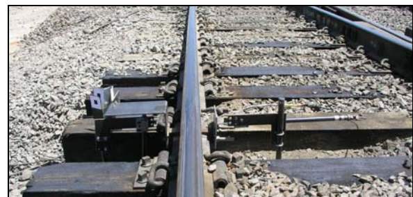
Figure 3. LVDTs used for Ground-Reference Measurements of Vertical and Lateral Displacement in the Frog Area under Traffic
