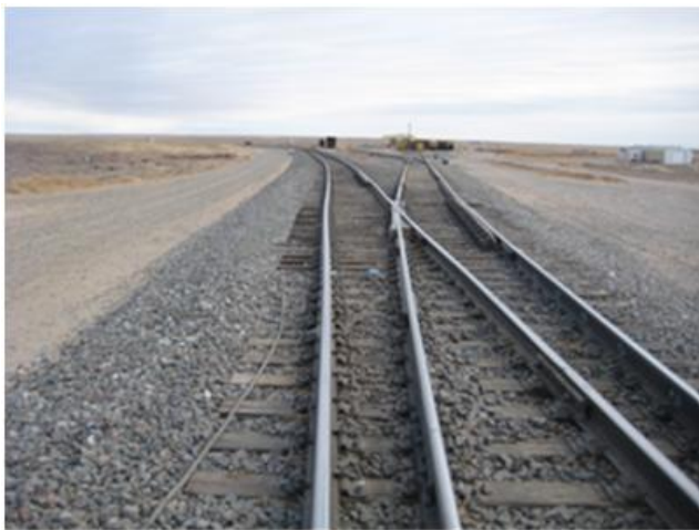
Figure 3. View of FAST No. 11 Lift Frog Mainline Alignment Deviation
