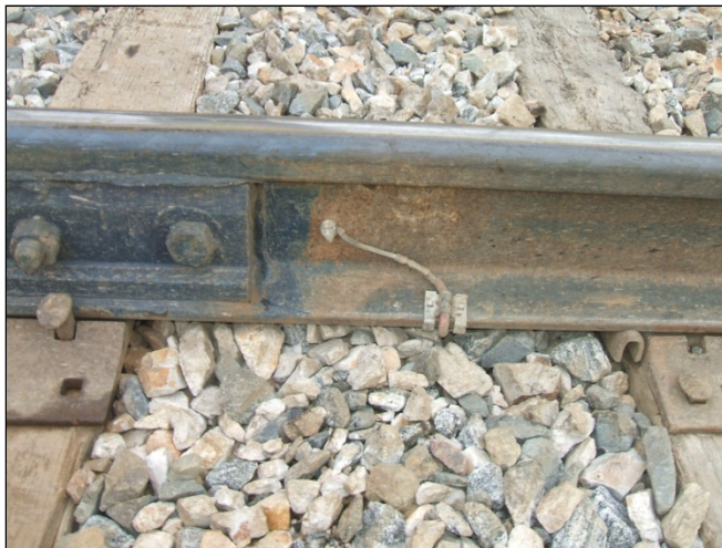
Figure 7: Example of Damage Resistance Installation on KCS, Where Wire is Routed Under the Rail and Buried in the Crib, Limited Snagging or Other Damage from Passing Vehicles and Maintenance Equipment (Note: Small clamp on rail base holds wire in position.)
