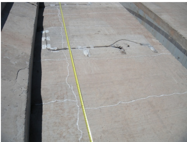
Figure 7. Post-Test Cracks in High-Rail Span Piece
