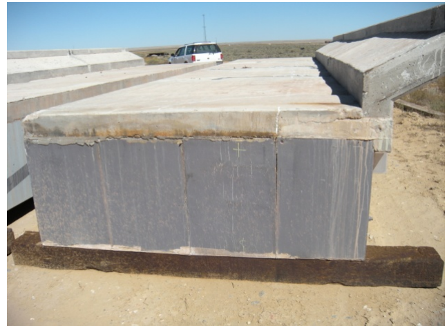
Figure 8. Cross Section Cracks in High Rail Span Piece
