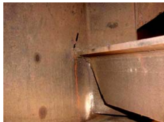
Figure 3. Crack in Web near Bottom Lateral Brace Connection, Inside of 55.5-foot Welded Girder
