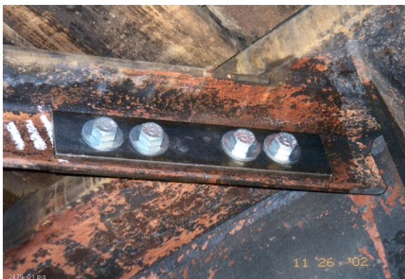
Figure 5. Typical Bolted Splice Repair of Broken Top Lateral Brace in 65-foot Welded Girder
