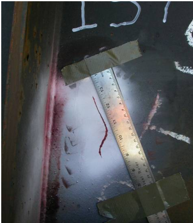
Figure 4. Crack in Web near Bottom Lateral Brace Connection, Outside of 55.5-foot Welded Girder
