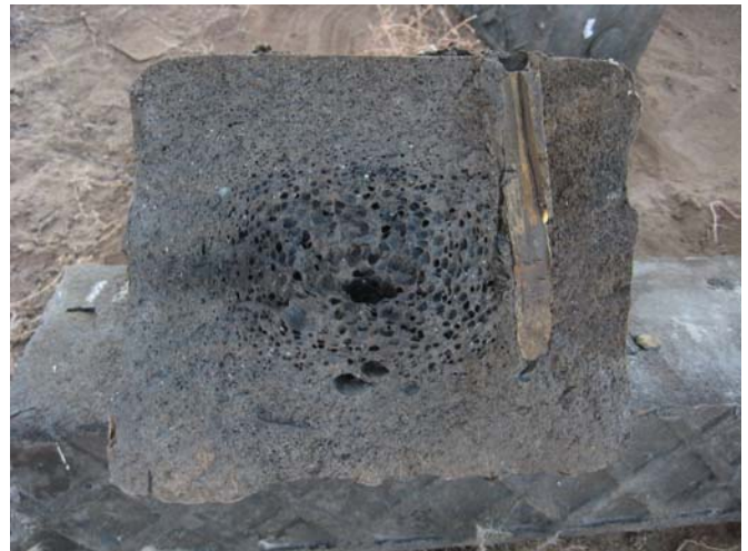
Figure 6. Tie Tek Plastic Composite Tie broke due to Wedging Force of Driving Spike and Very Hard Plugging Material
