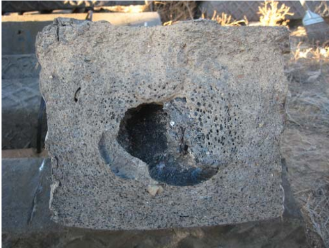
Figure 5. Tie Tek Plastic Composite Tie broke at a Material Void near its Center
