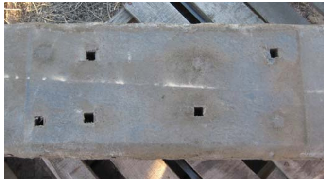
Figure 7. Tie Tek Plastic Composite Tie with Minimal Damage in Tie Plate Area and Minimal Deformation of the Cut Spike Holes
