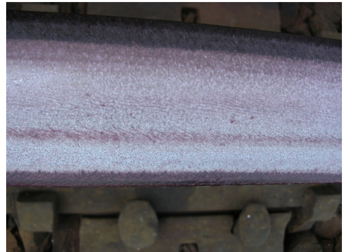
Figure 10. Low Rail of Curve D in the non-TOR Treated Zone at Site 5. End of Test June 2009
