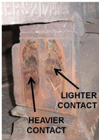
Figure 5. Indication of Uneven Pressure on Column Wear Liners
