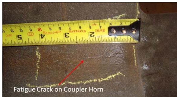
Figure 6. 3.5-inch Fatigue Crack on Coupler Horn
