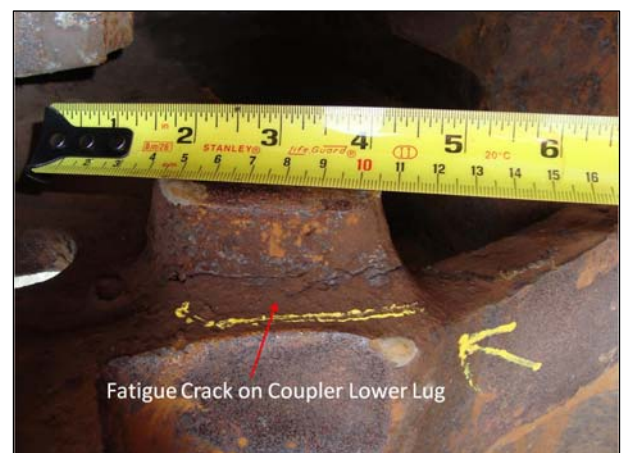
Figure 8. Fatigue Crack on Coupler Pulling Lug
