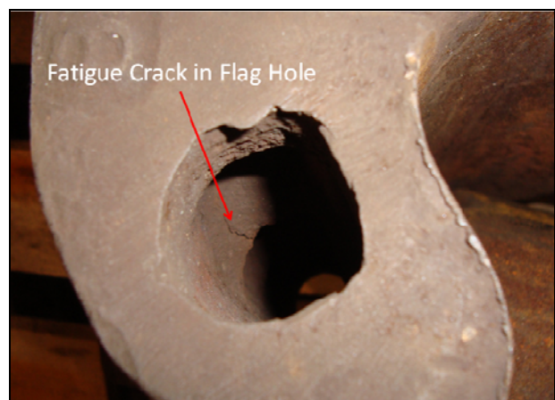
Figure 9. Fatigue Crack in Flag Hole of Knuckle
