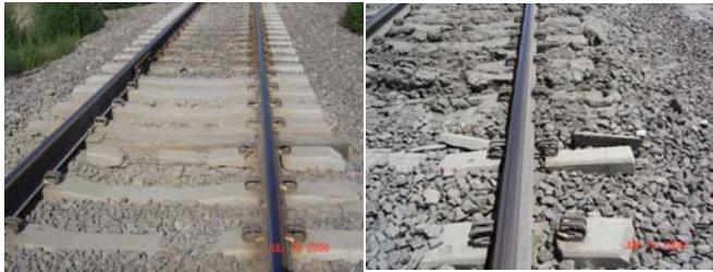
Figure 1. Example of Track Degradation on a Ballasted Deck Concrete Bridge
