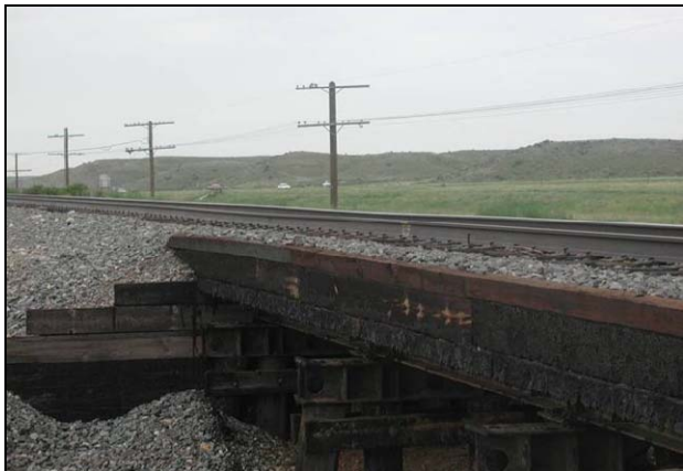
Figure 2. Track Surface Low Spot on the Approach to a Ballasted Deck Bridge
