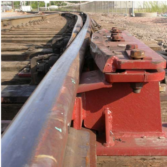
Figure 1. Typical Field Side Switch Point Guards
