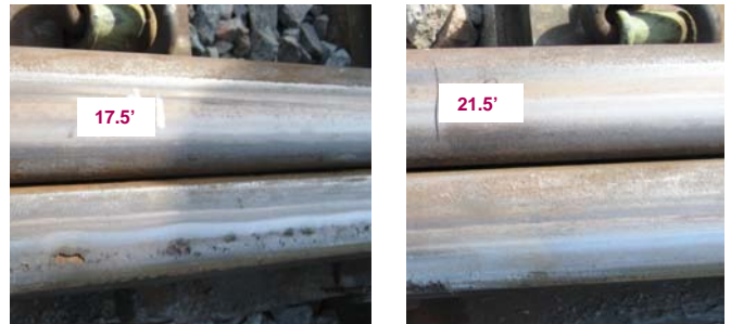
Figure 4. Rail Surface Conditions versus Distance from the Switch Point Tip (Diverging Route)
