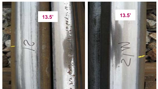
Figure 5. Surface Condition of the Switch Rail and the Matching Stock Rail at the Same Distance from the Switch Point Tip
