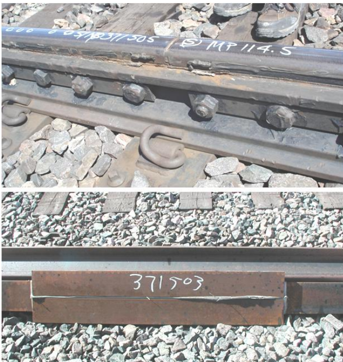
Figure 4. An IJ with Wraparound Joint Bars (top) In Service, (bottom) View of the Rail Base
