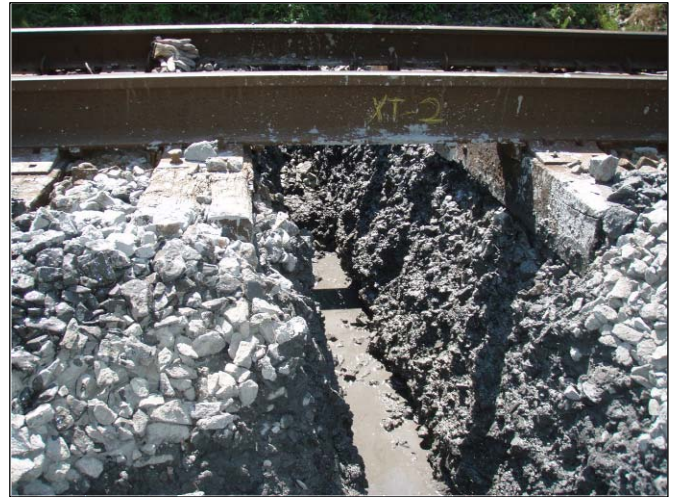
Figure 4. Water Collecting in the Bottom of XT-2 Trench
