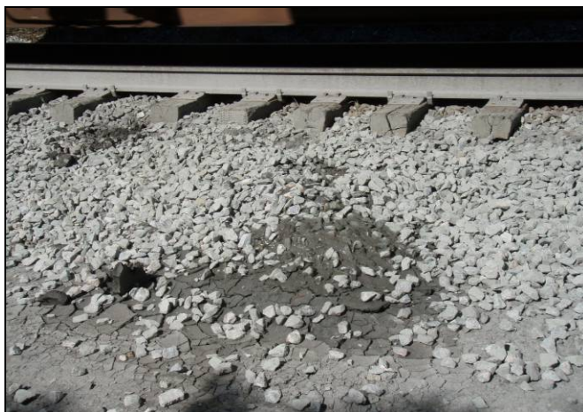
Figure 7. Mud Pumping through Ballast Shoulder at Site 3
