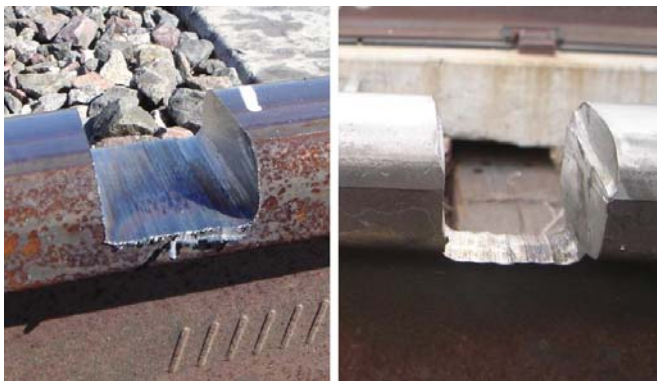
Figure 1. Ground Slots for Railhead Repairs. Railtech Boutet 1-inch Depth Slot (left) and Orgo-Thermit Full-Head Depth Slot (right)
