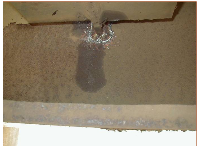
Figure 4: Treated Weld Detail between Beam and Cross-Frame Member
