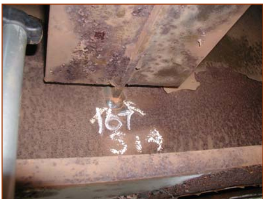
Figure 9: Crack in Weld above a Previous Crack in Span 14
