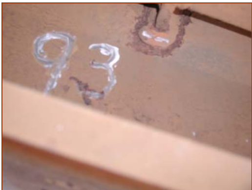
Figure 8: Crack in Weld above Treatment Application in Span 10
