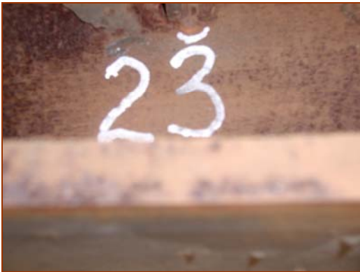
Figure 7: Crack in Partially Treated Weld in Span 6
