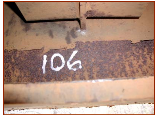
Figure 10: New Medium Crack on Previously Okay Detail in Span 10
