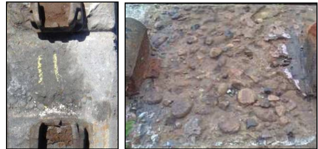
Figure 1. Examples of Rail Seat Deterioration 1
