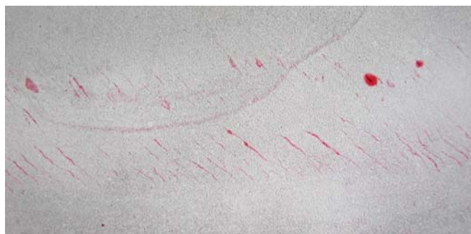
Figure 2. Example of RCF Cracks that Produced a Visible Result with Dye Penetrant Applied
