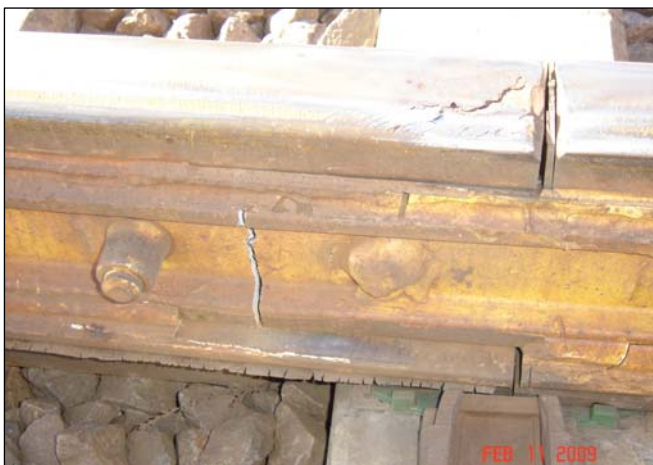
Figure 3. IJ Failed due to Crack Bar at 1,090 MGT
