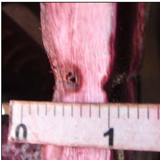
Figure 3. Porosity Defect Identified using Liquid Penetrant Inspection
