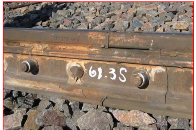
Figure 6. Cracked and Replaced Joint
