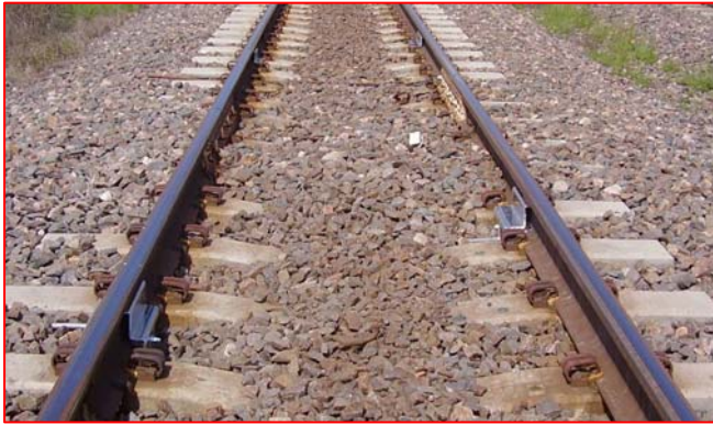
Figure 3. RNT Sensors Installed at Test Site
