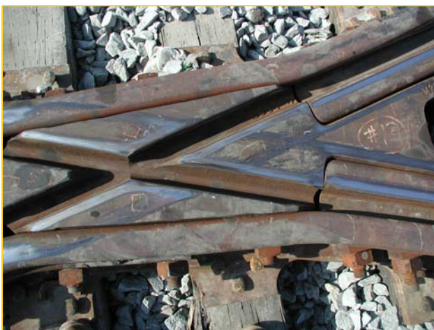
Figure 1. Running Bands on a New Frog Flat Rail Surface
