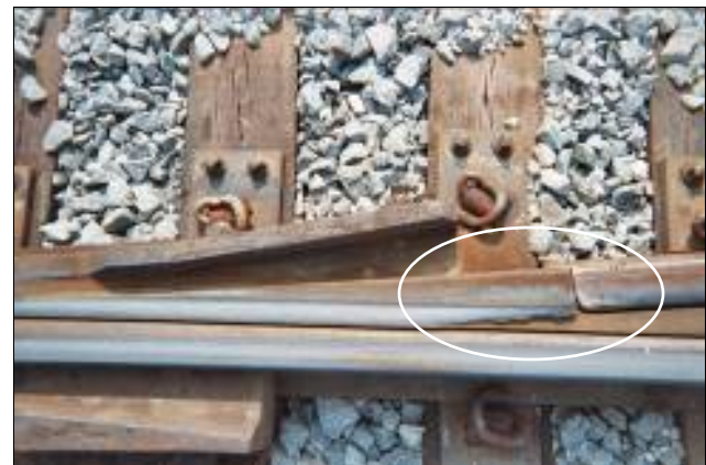
Figure 5. Metal Flow on Frog Heel Mainline Easer Ramp
