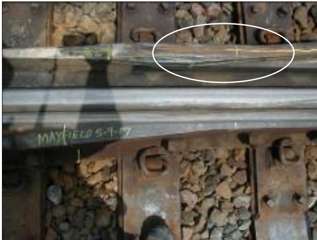
Figure 6. Mainline Rail Wear due to Crossing Wheels
